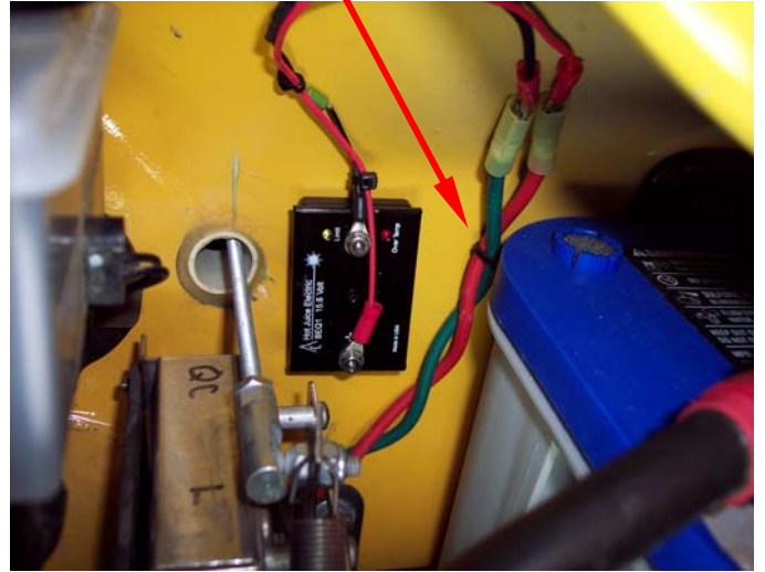
Battery #6 installation Connect BEQ1 leads to access lead. Red wire is Positive. Secure wires with Gaffers tape as shown below.
