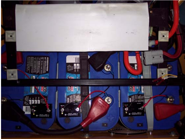
Batteries 7, 8, and 9 installation
