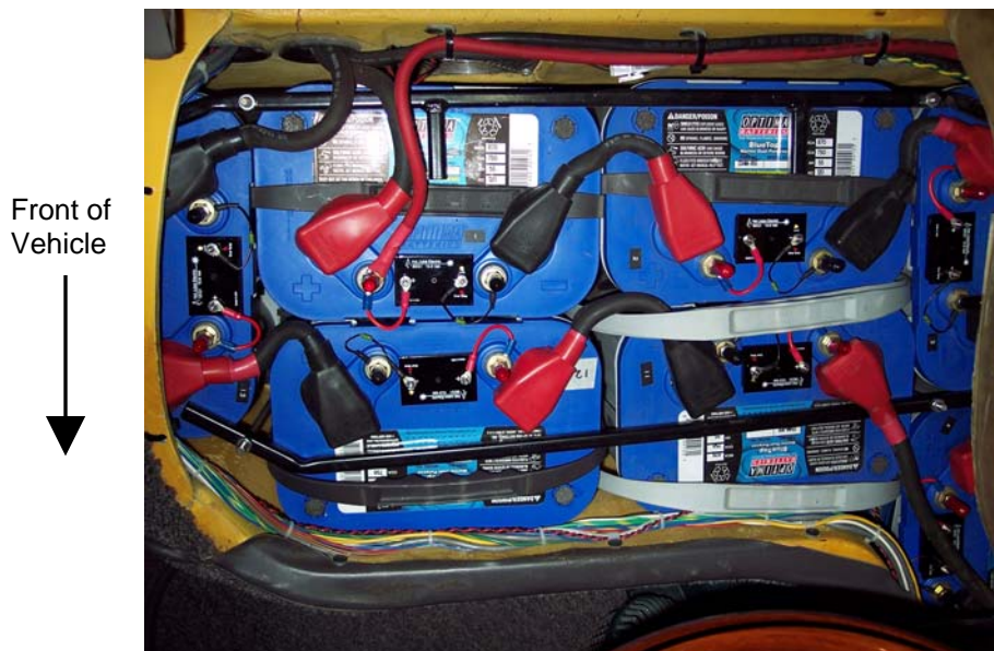
Under seat installation Batteries 1, 2, 3, 4, 11, 12, and 13.
